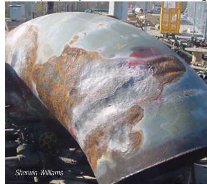
FIGURE 2. Heat-cycling is an important factor in causing CUI, because it can lead to condensation, which introduces moisture into the corrosion zone at the component surface
