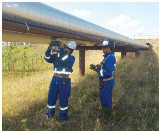
FIGURE 4. Technicians use non-destructive testing to detect the presence of moisture, an indication of where CUI may be a problem
