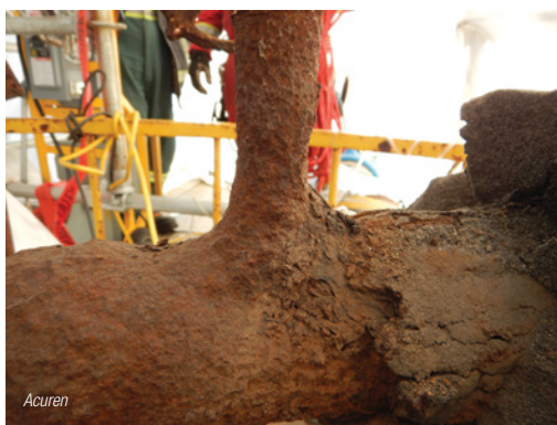
FIGURE 1. Corrosion under insulation (CUI) is a phenomenon that can be particularly aggressive when the presence of moisture is combined with contaminants at a steel surface, and so it can progress rapidly between asset inspection intervals
